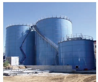
Anaerobic Digester Tanks
