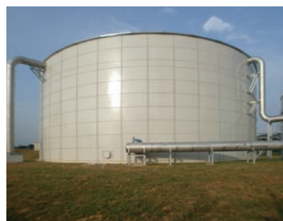
Potable Water Storage
