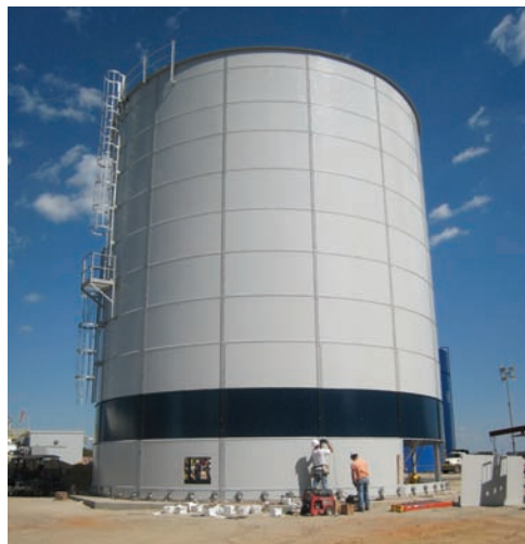
Power Utility - Process Water
